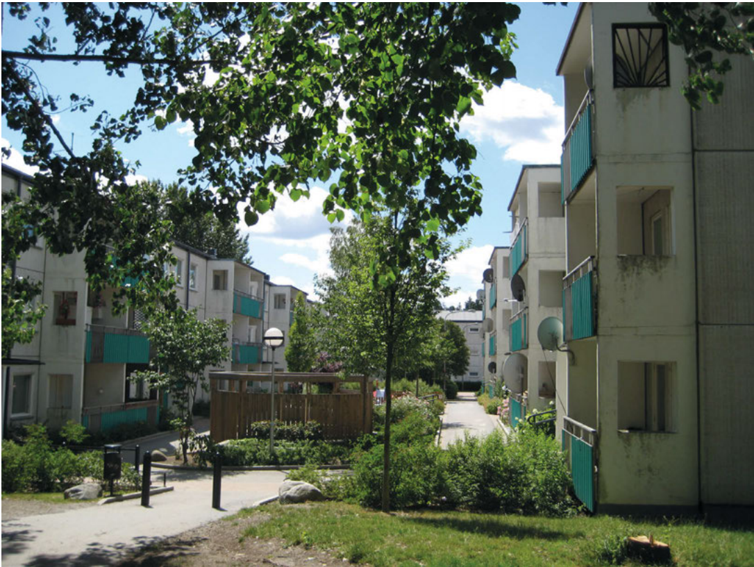
Some facades in Tensta stay intact, although exposing the varying quality and durability of the prefabricated building elements. Still, the environment of this courtyard is intimate and green like in Vällingby.
